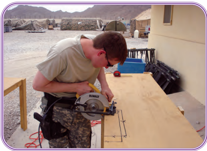
Specialist Ronnie M. Heflin build shelves for the medical supply room at the hospital. The SORT laboratory technician, Heflin applied his carpentry skills to improve the “bare bones” facility.
